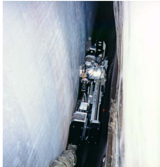
Navigator at Chin Shan Unit 2 traveling between the reactor vessel OD and mirror insulation
